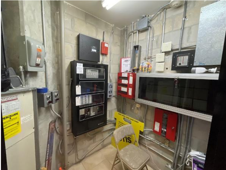
Photos / Fire Protections
