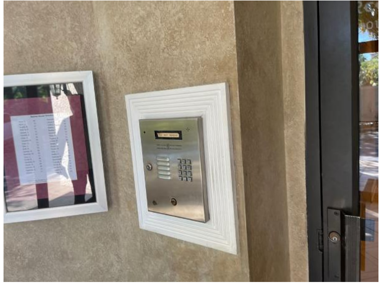
Photos / Fire Protections
