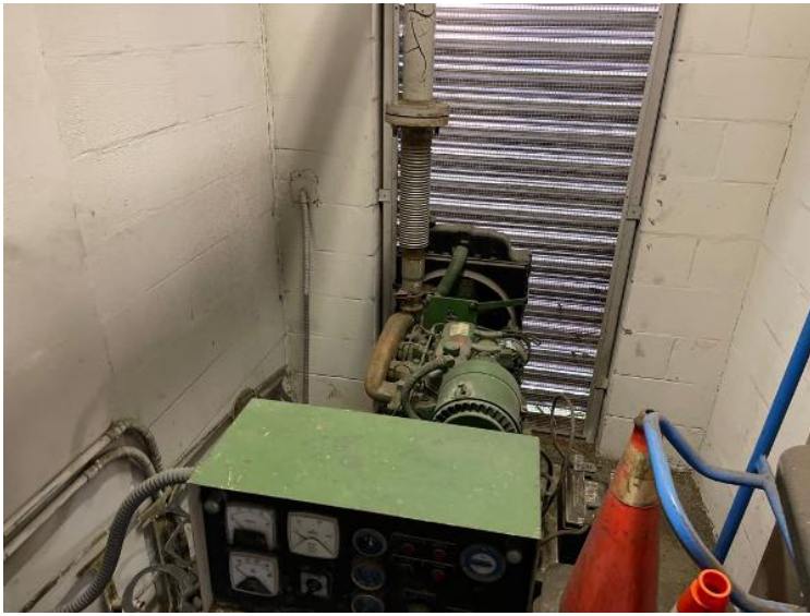
Photos / Fire Protections
