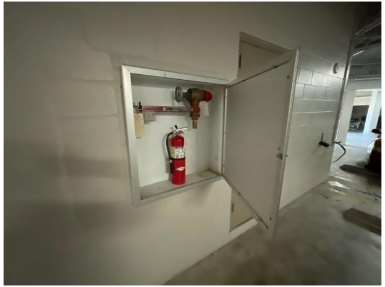
Photos / Fire Protections
