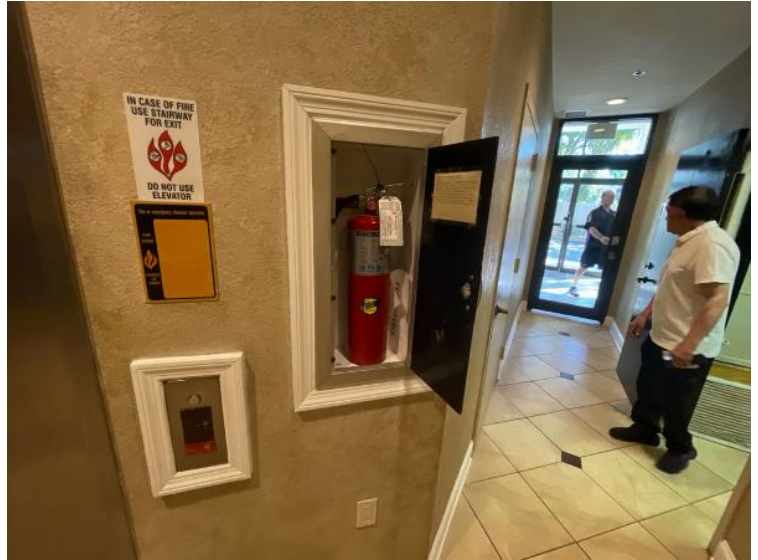
Photos / Fire Protections
