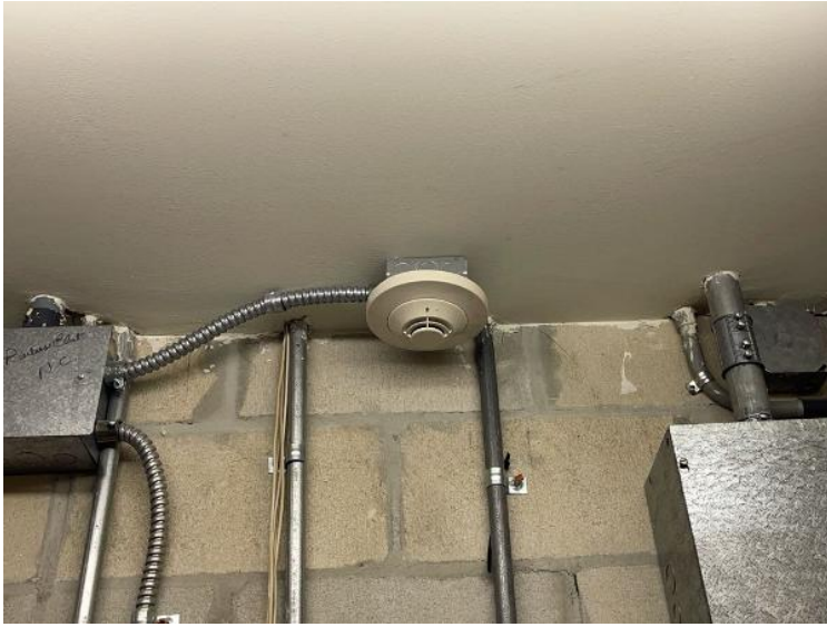
Photos / Fire Protections
