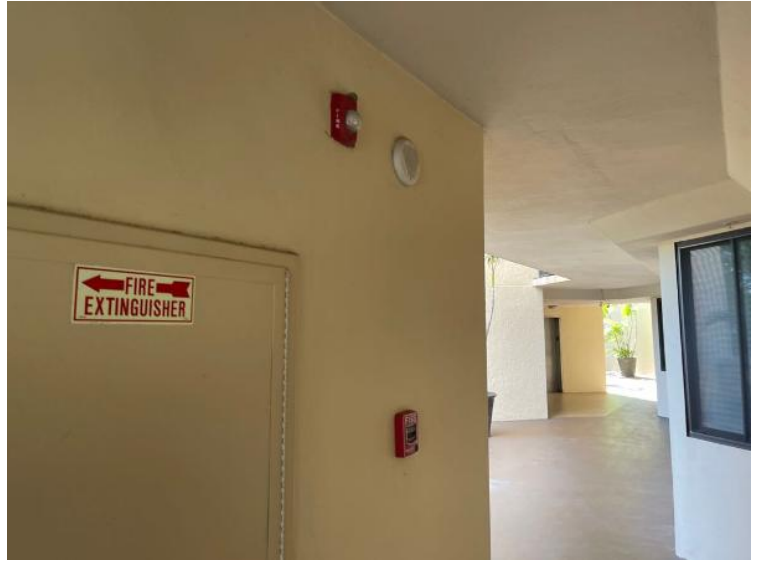
Photos / Fire Protections
