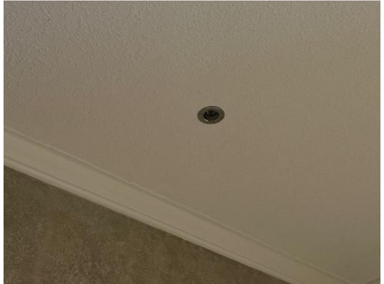
Photos / Fire Protections
