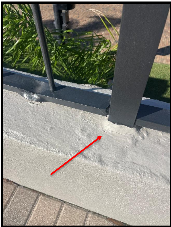
Minor cracks at post pocket
