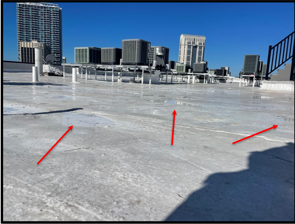
Areas with minor water ponding
