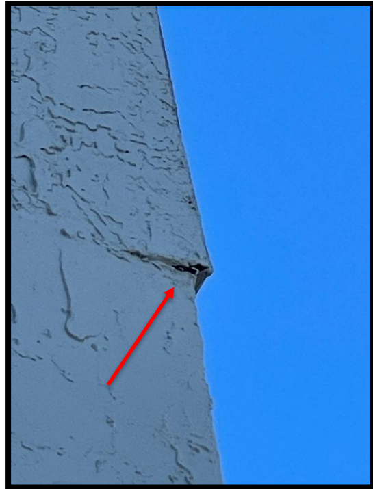
Small breach in Stucco Façade
