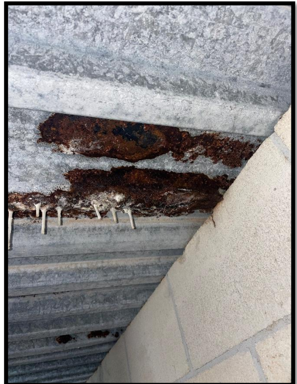
Corroded areas on metal pan and ribs
