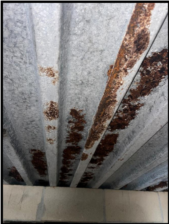
Corroded areas on metal pan and ribs
