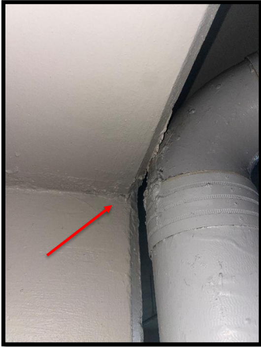
Recent touch-up on tie-beam
