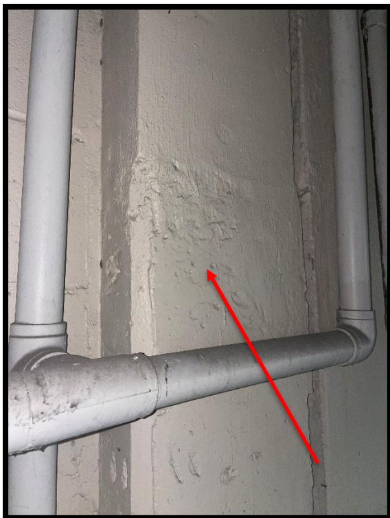
Minor spalling on concrete substrate
