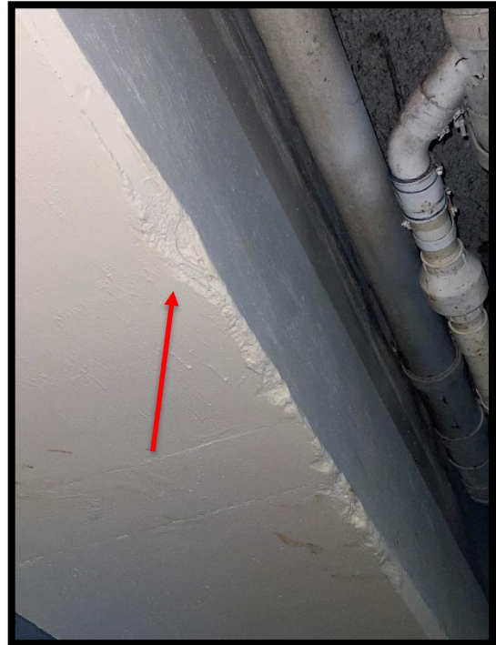
Minor spalling on tie-beam
