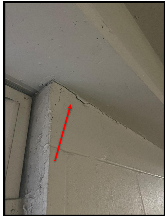
Separation crack @ perimeter wall
